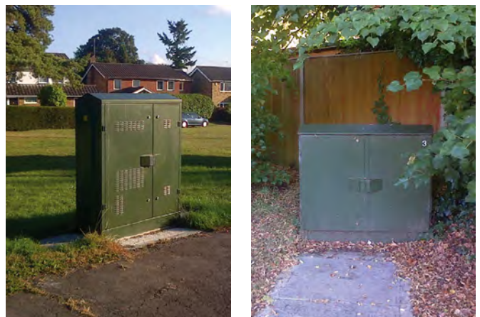
Fig 9.2: The telecommunications box on the left is sited so as to appear very prominent, whereas the box on the right has been located more sensitively near a fence (rather than in open space) and its appearance is softened by surrounding vegetation.
