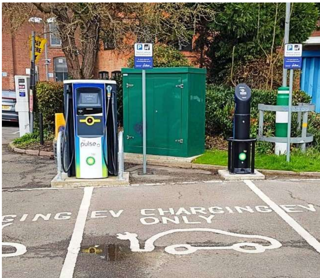
Electric Vehicle Charging points in Chesham
