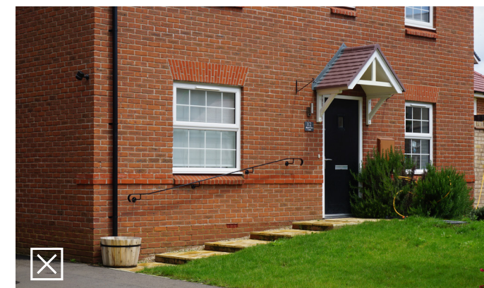
Access to property is made difficult by poor response to site levels
