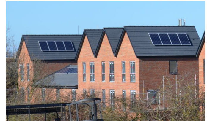
Solar panels at Brooks Mews, Aylesbury
