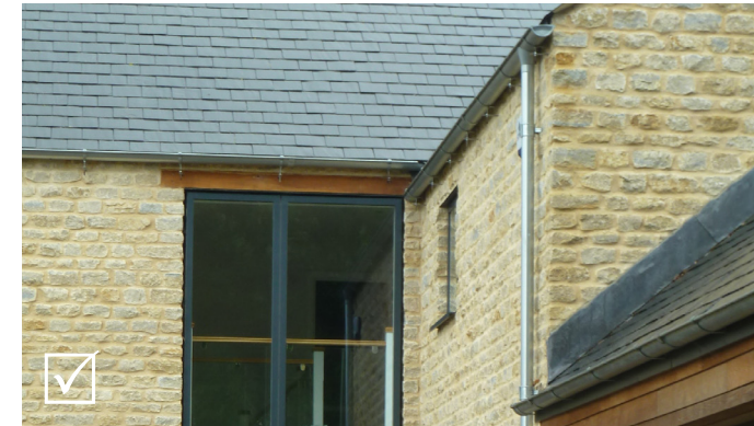
Rain water pipes have been positively accommodated using high quality materials
