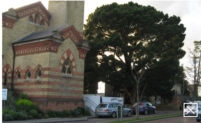
Entrance to nursery is not designed to be respectful of the historic chapel
