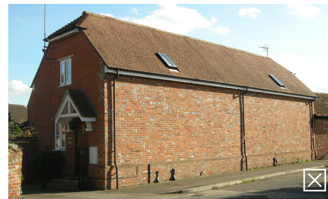
Domestic style porch and projecting roof lights detract from the barns character
