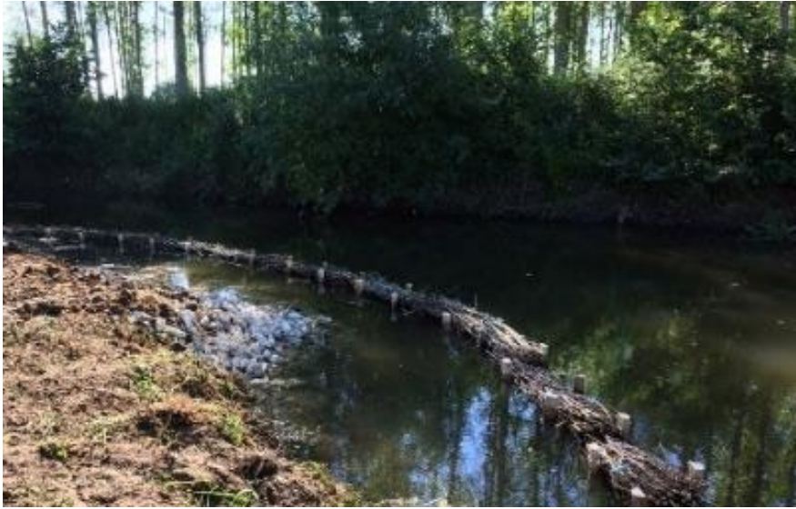
Photo 5: Willow spilling is an example of a soft engineering technique to support and improve watercourse bank stability. Photo credit: River Thames Conservation Trust.
