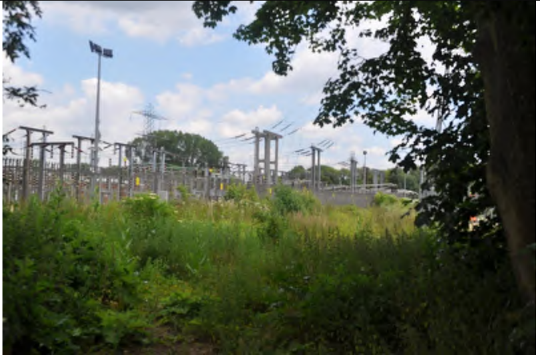
Photograph 1: Electrical sub-station in the south-east corner of General Area 79.
