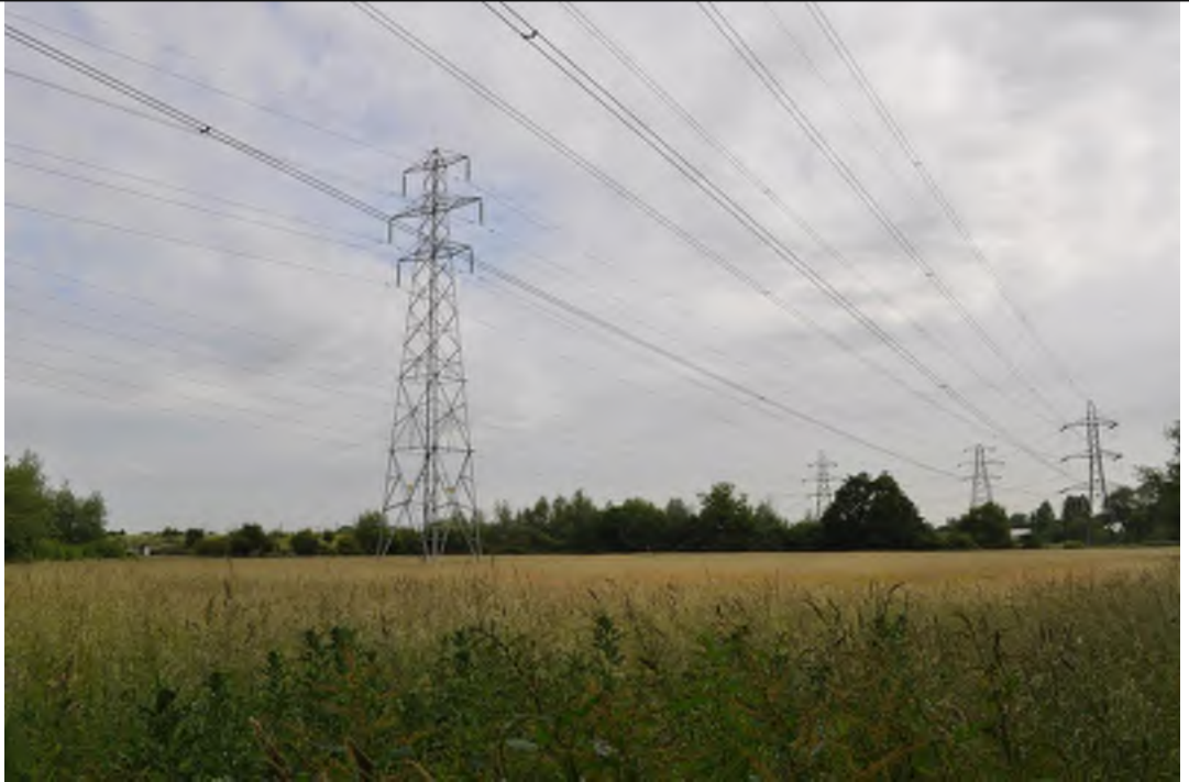
Photograph 1: Looking north-east from Palmers Moor Lane, in the east of General Area 83.
