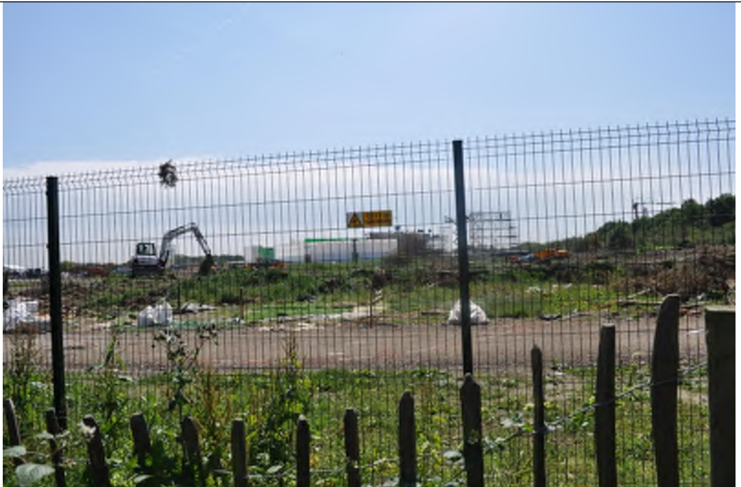
Photograph 2: Construction at the expanded Pinewood Studios site, south of Seven Hills Road.
