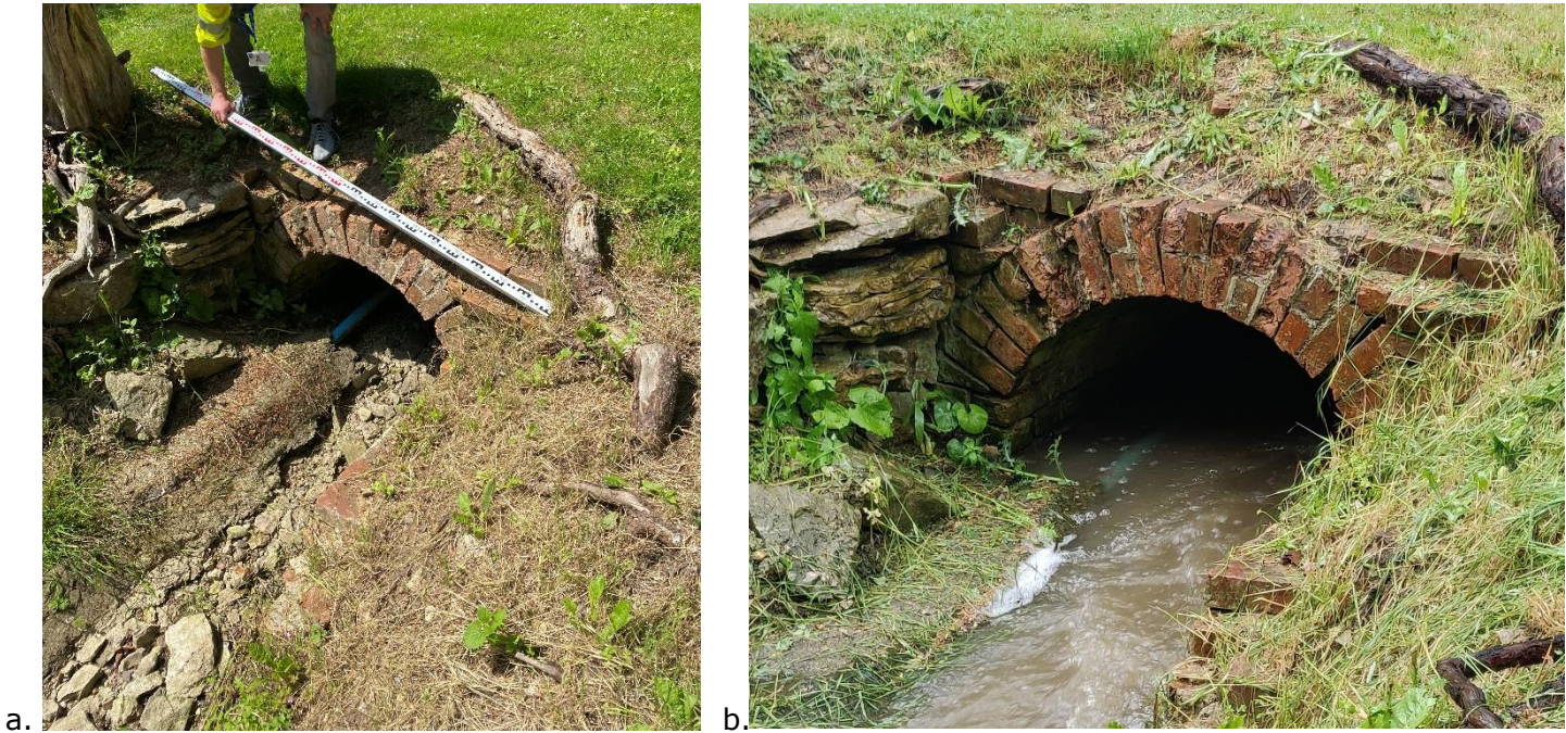
Figure 10-3: Channel condition at the School Fields culvert inlet, showing channel modifications, with no flow on 02 July (a); and with flow on 18 June (b).
