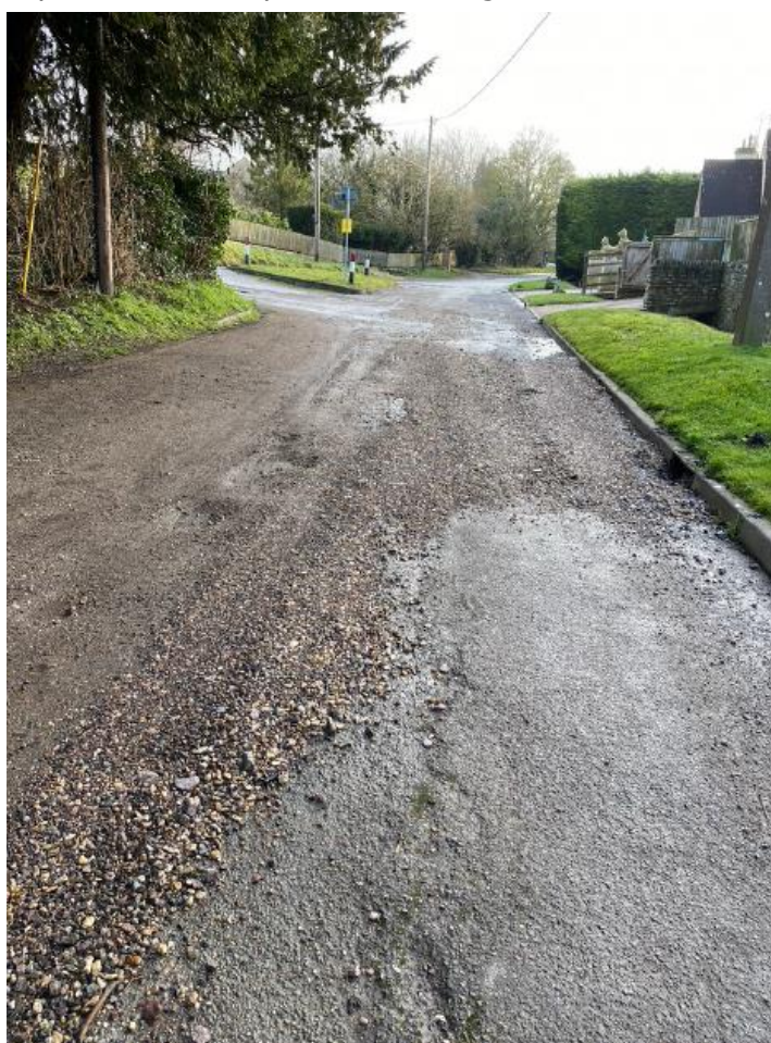
Figure 8-6 Sediment deposited on road near Bridge Cottages
