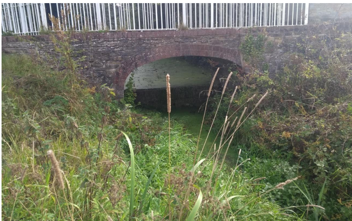
Figure 9-2: Tonne Brook on High Street (pond outlet), September 2021.
