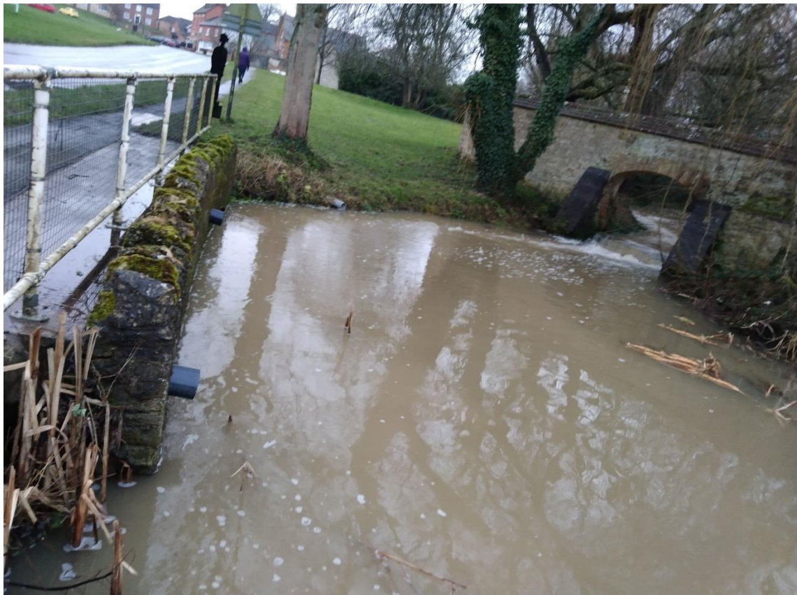
Figure 8-6: The inlet to Thornborough Pond at time of high flow. Credit: Thornborough residents
