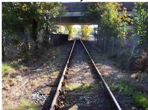
The railway is raised only slightly above the level of roads to either side
