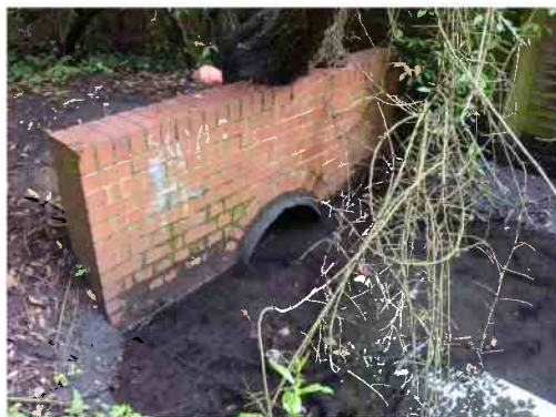
The Newt Ditch culvert at its outfall was observed to be heavily silted
