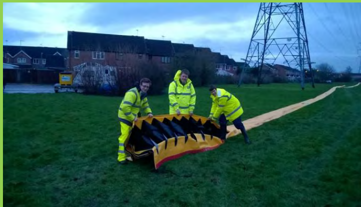
BCC Strategic Flood Management Team deploy a length of the flood barrier at The Willows
