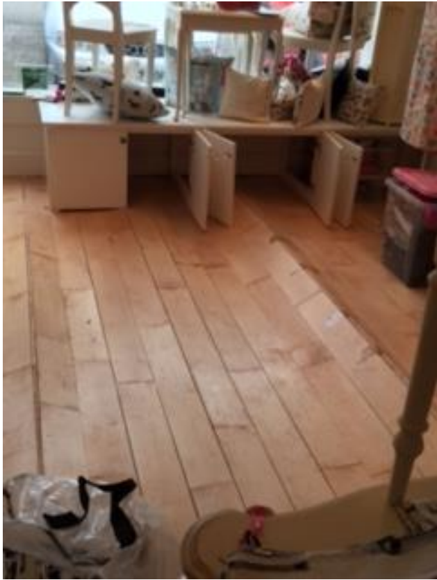
Internal flood damage to a business on High Street, Old Amersham
