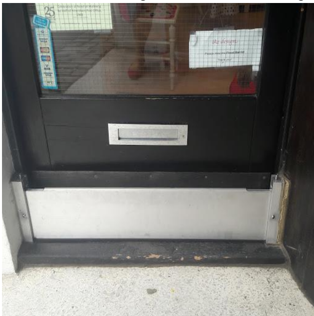
Property level protection installed as a result of the event (Anastassopoulos, 2017)
