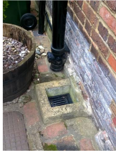
Drain outside property on High Street
