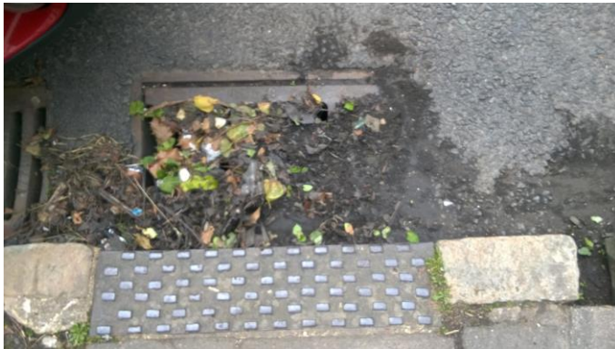
High street drains post event
