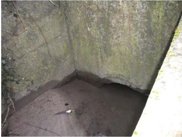
Figure 9 Silted up gully at Stratford Drive (Chris Spreadborough, Resident)
