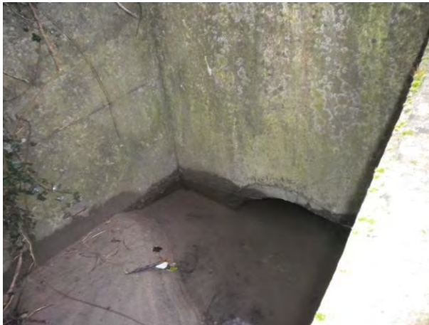
Silted up gully at Stratford Drive
