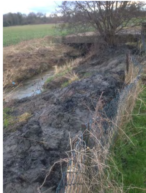
10/02/2014 16:52 Silt removed from Stoke Brook and gully outfall at end of Fox Glove - Councillor Steven Lambert
