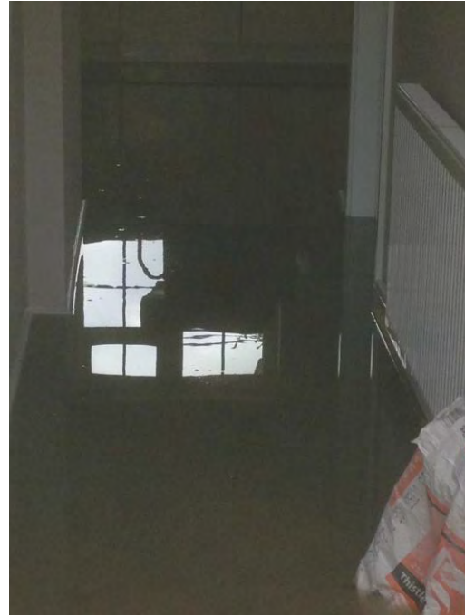
07/02/2014 12:27 Internally flooded property - Councillor Steven Lambert
