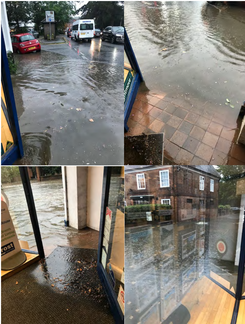
Figure 2, 3, 4 and 5 – Photos of flooding taken by the Frost Partnership on 24/09/2019
