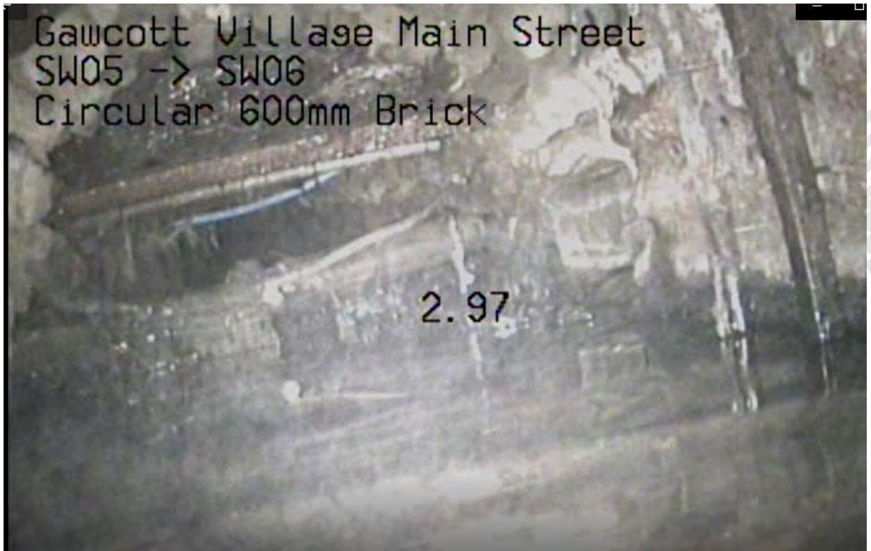
Figure 9-3: CCTV survey - several pipe crossings through culvert
