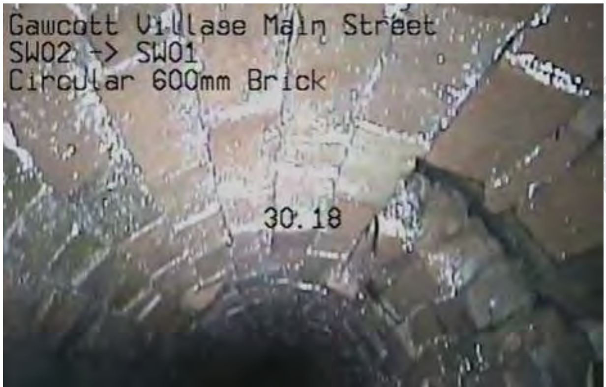
Figure 9-1: CCTV survey - hole in wall of culvert
