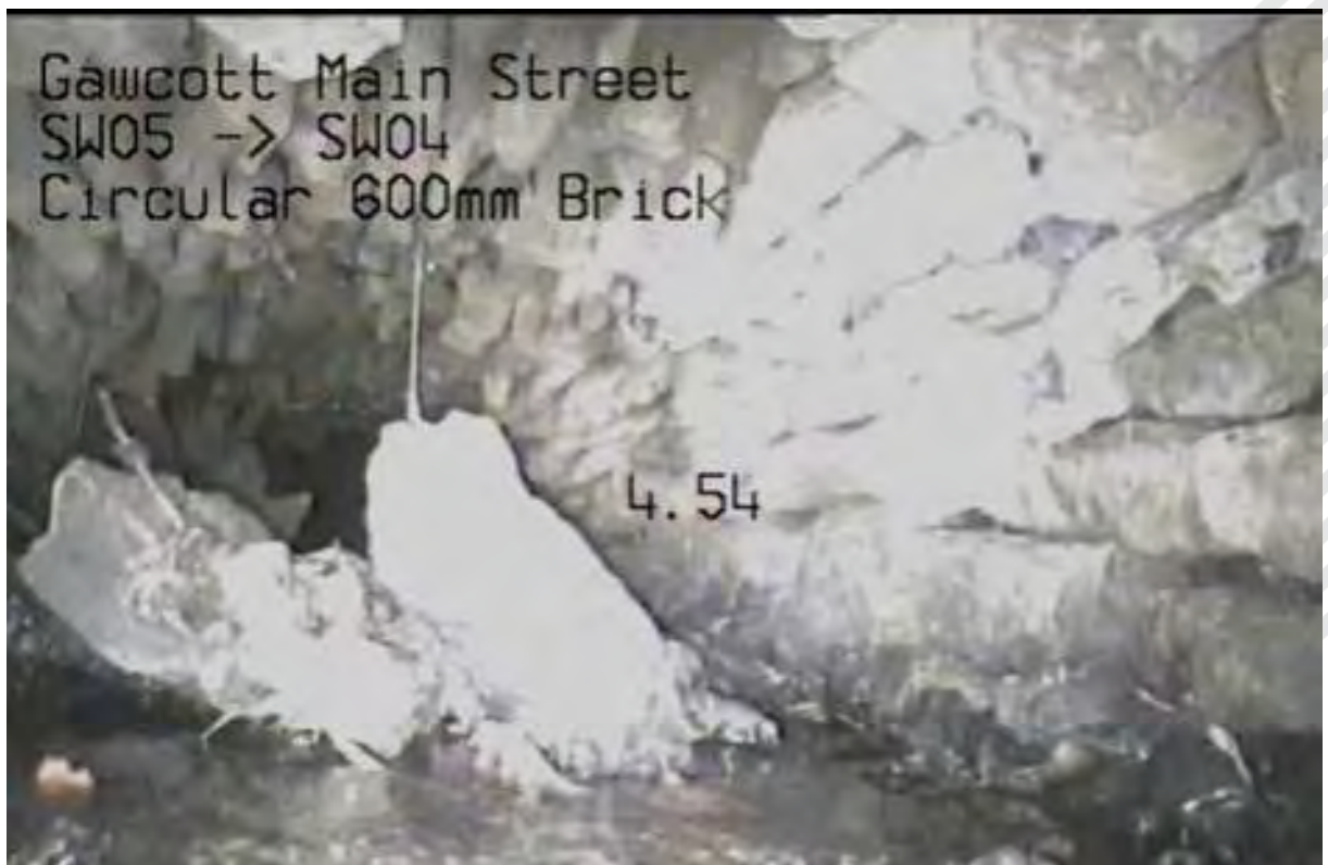
Figure 9-2: CCTV survey - masonry in base of culvert, 40% blockage.
