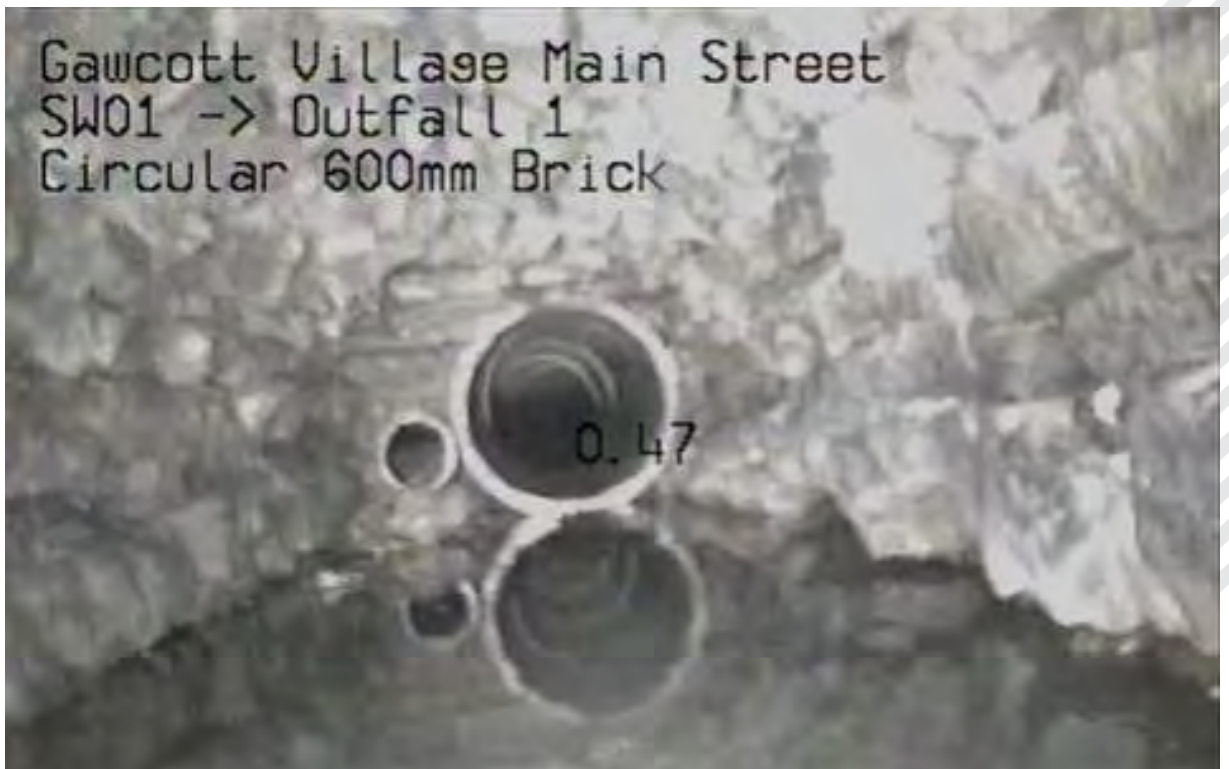
Figure 9-4: CCTV survey - change in culvert size from 600mm to 150mm and 300mm
