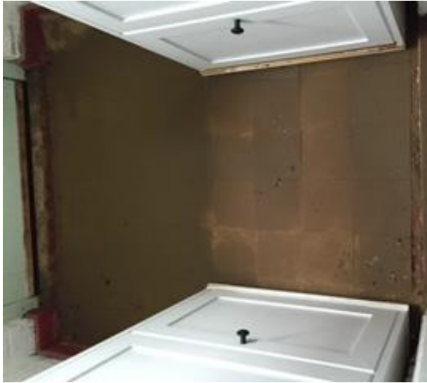
Figure F14: Silt in hall way Rignall Road May 2018
