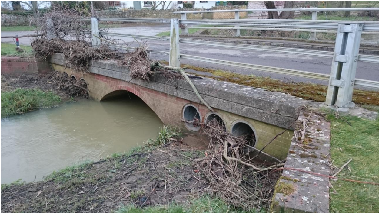
Figure 10: Debris build up on South End bridge at east of village, 11 th March 2016 (photo by BCC).
