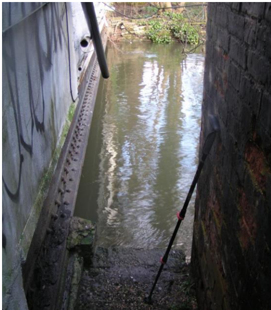
P1010143 TQ0504084755 Looking NE low bank level Showing the low bank compared the opposite bank and bridge soffit.
