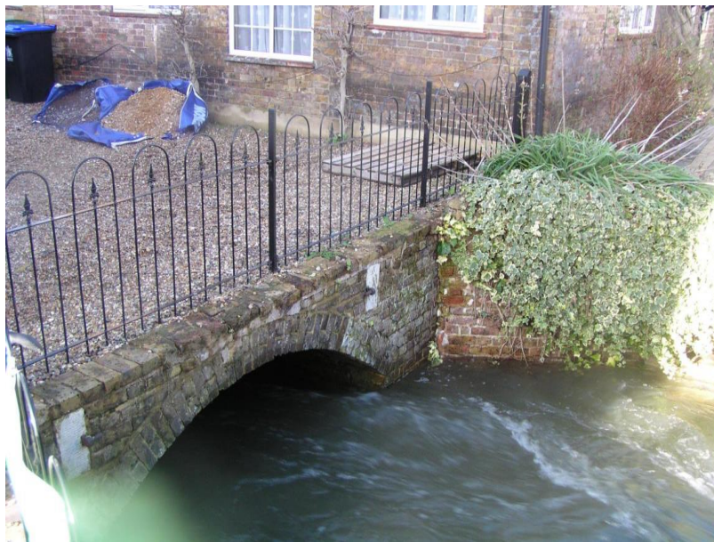
P1010154 TQ0510884741 Looking N culvert exit w-l Water level in the channel by Mill Stream Cottage.
