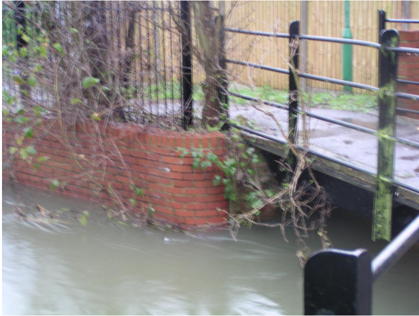
P1010104 TQ0497484861 looking E channel w-l Water level at the footbridge by Alder Road, 11 courses of bricks from the top of the wall.
