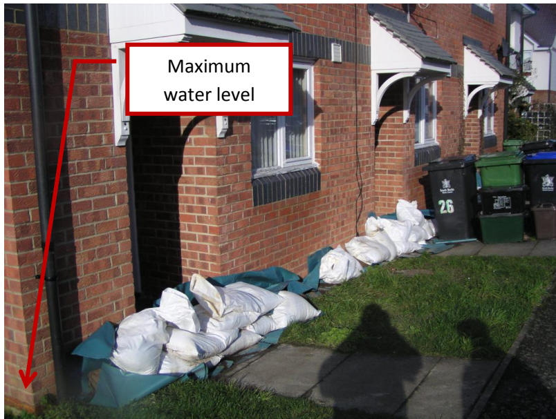
P1010133 TQ0491785087 Looking NE 25-27 Oakside Sandbagging to properties that came closest to flooding internally. Water level marked with yellow crayon in bottom left corner.
