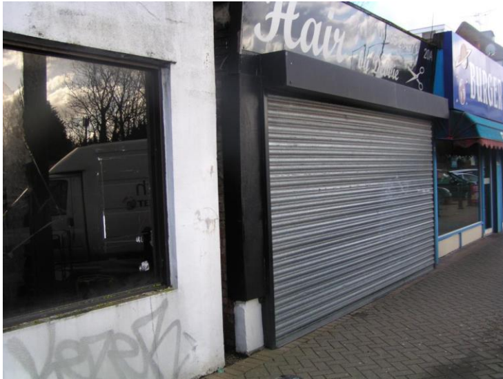
P1010140 TQ0503584750 Looking E 20a Oxford Rd The gap beside the hair salon through which flood water flowed.
