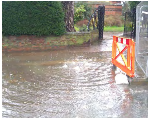
Surcharging manhole, High Street. Photo courtesy of CSP Parish Council, 16/03/14
