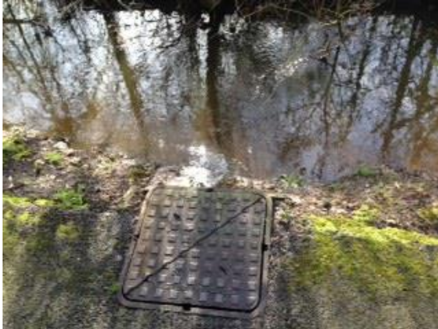
Surcharging combined sewer (Tingdene Park Homes, 10 th February 2014)
